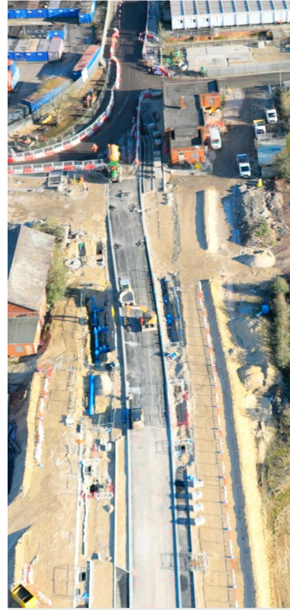
The new link road connecting into the top end of existing Leeman Road
